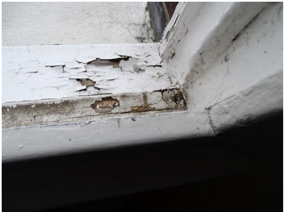
Bedroom 1 bottom sash frame rotten
