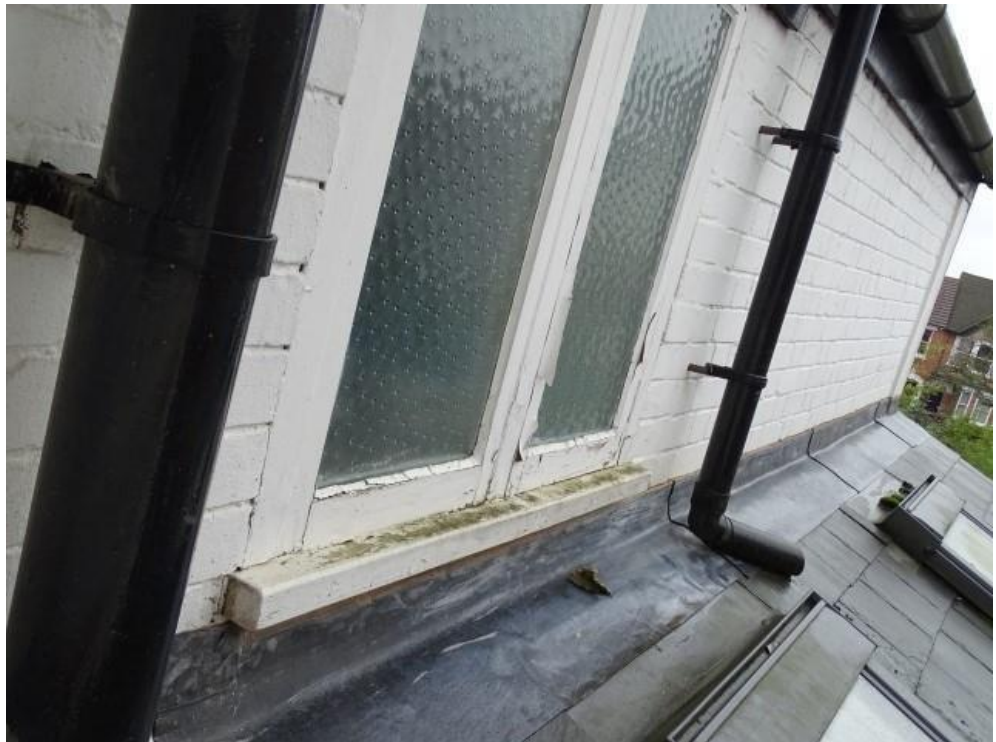
Bathroom fixed casement rotten
