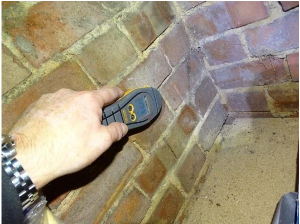
Wet wall in loft above bedroom 3
