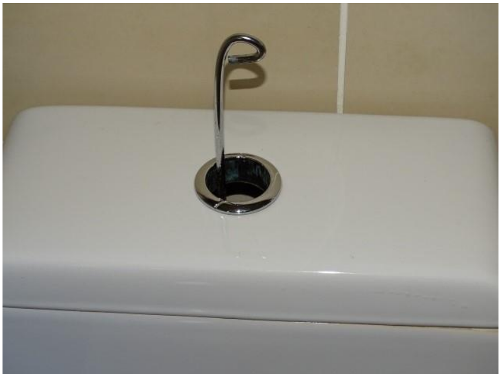
Flush mechanism button broken
