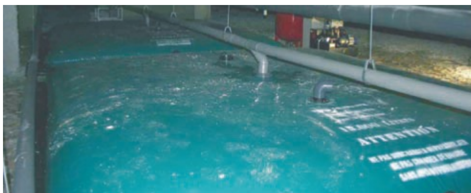
2 x 15 m 3 internal rainwater recovery
