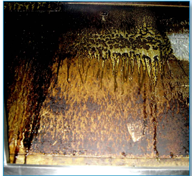
Behind Grease Filters in Canopy Before Cleaning
