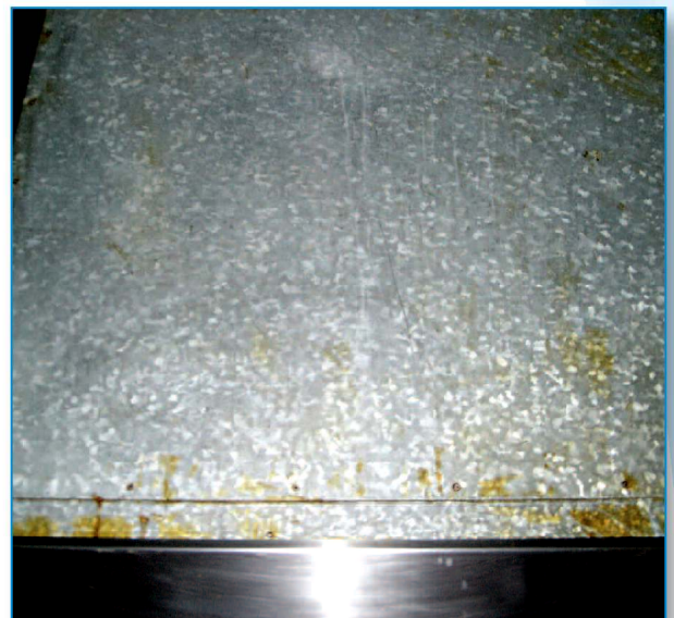
Behind Grease Filters in Canopy - After Cleaning
