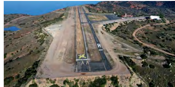
Catalina Runway 4/22 will be a temporary runway for limited flights until mid-April, when the new concrete runway is expected to receive its first flight.
