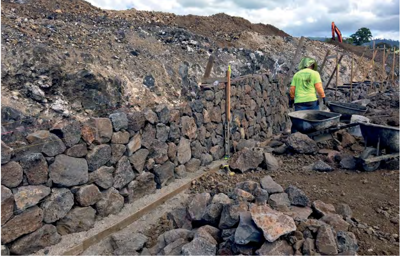
Reused rock found at the Makali'i at Wailea project site being used to build walls.
