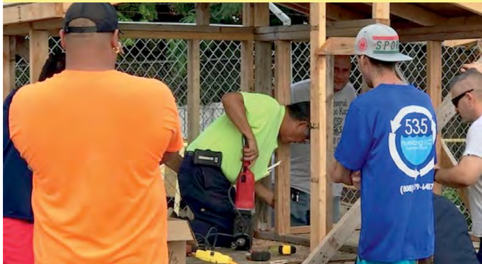
Plumbing instructor Maurice Torigoe (center) explains rough-in steps for sewer, waste and vent piping.
