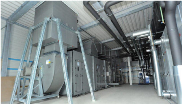
Air Handling Units installed at a large university fume cupboard exhaust system. Constructed entirely from Polypropylene offering excellent chemical resistance.
