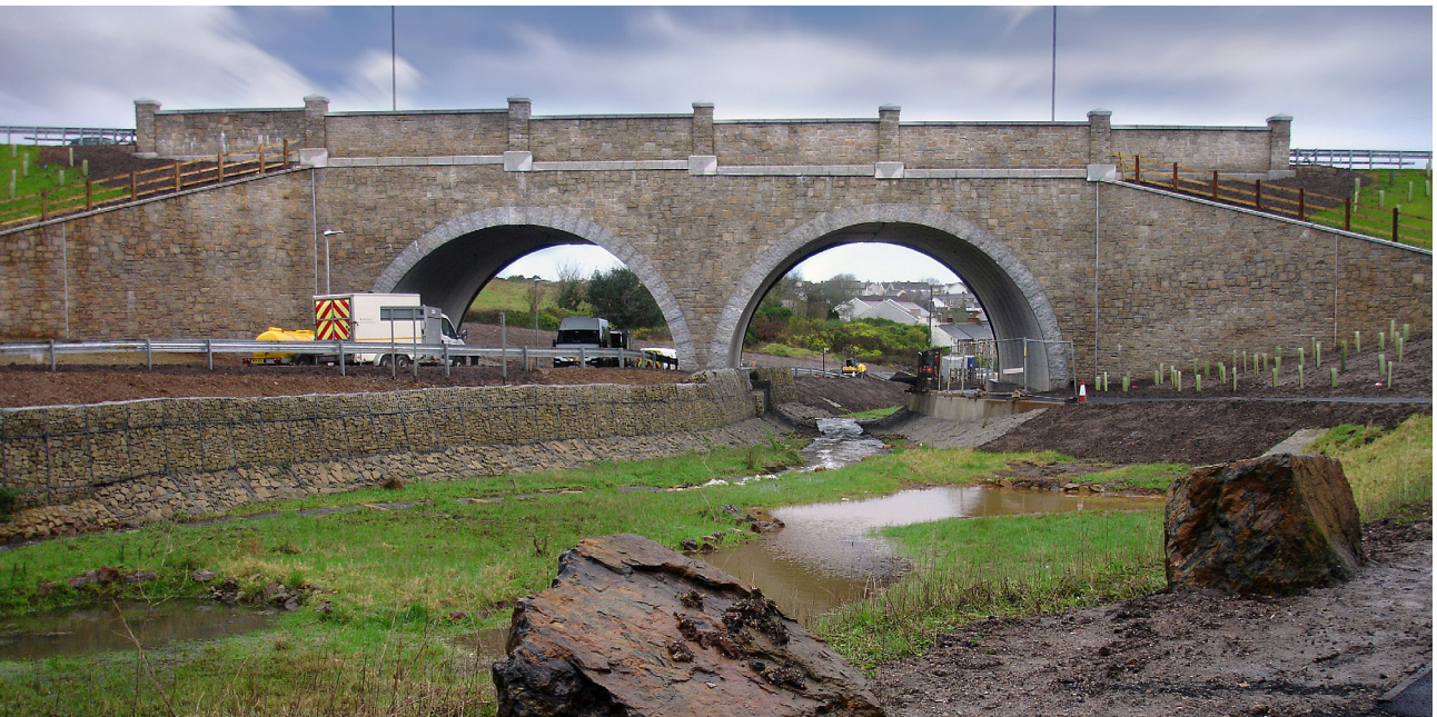
Camborne Pool - Redruth East - West Link - Red River Valley Arches (asset BEBO® Twin Arches C42T/5 - Span 12.802m - Rise 6.807m)
