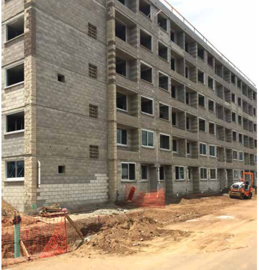
Mitsunaga Construction builds Kahului Lani in Kihei. PHOTO COURTESY STEPHAN KEALOHA/CATHOLIC CHARITIES HAWAII
