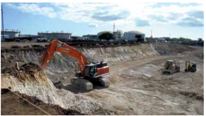
Nan Inc. is GC on the city's $267.2 million Honouliuli Waste Water Treatment Plant. PHOTO COURTESY NAN INC.
