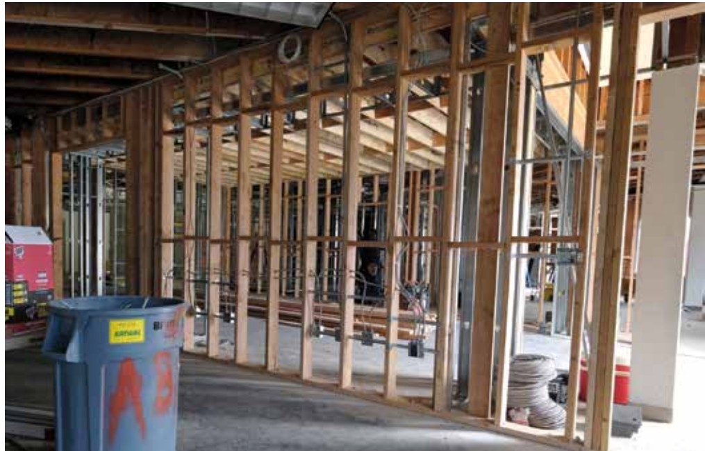
Arisumi remodels the Liliuokalani Trust Children’s Center. PHOTO COURTESY MICHAEL BISSELL/ARISUMI BROTHERS INC.
