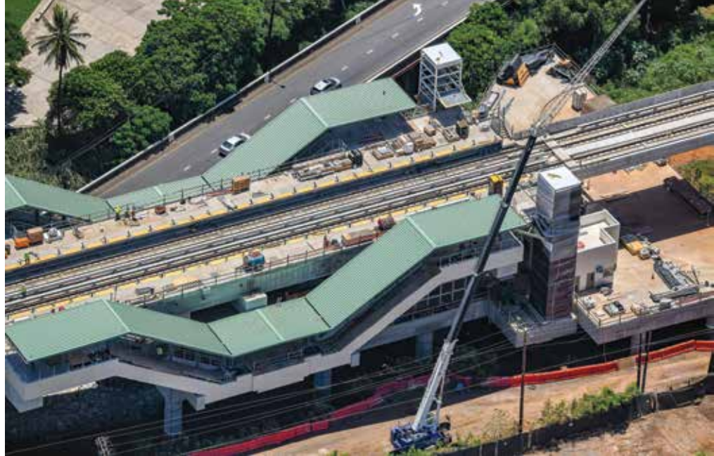
HART's Waiawa-Pearl Highlands Station, built by Nan Inc., is 80 percent complete. PHOTO COURTESY HONOLULU AUTHORITY FOR RAPID TRANSPORTATION
