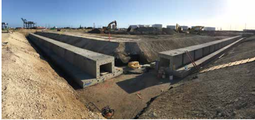
Kiewit has installed 1,200 linear feet of box culvert at the KCT Phase I. PHOTO COURTESY KIEWIT INFRASTRUCTURE WEST CO.
