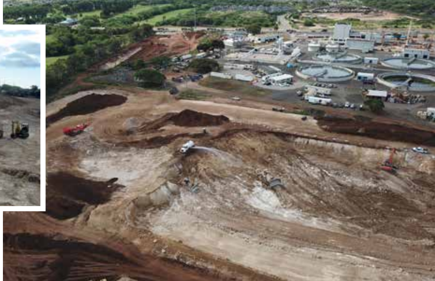
Nan Inc. Phase 1B construction at Honouliuli includes an aeration basin and six clarifiers, among other key features. PHOTO COURTESY NAN INC.
