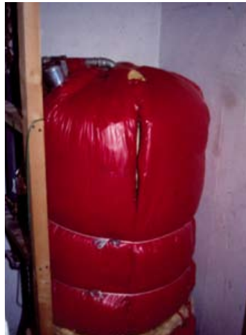
Figure 19 Domestic hot water cylinder with asbestos removed, lagged with a non-asbestos jacket
