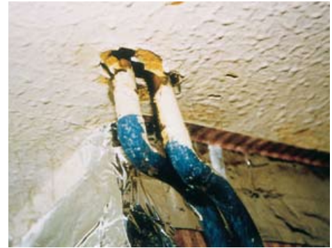
Figure 14 Decorative coating containing asbestos
