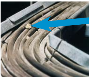
Figure 38 Asbestos debris in a cable tray
