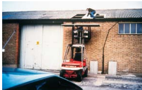
Figure 45 Work on a fragile asbestos cement roof without proper precautions
