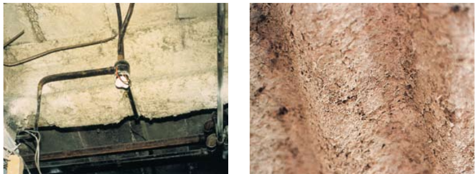
Figure 30 Distance (left) and close up (right) pictures of sprayed 'limpet' asbestos coatings. These can contain up to 85% asbestos which is loosely bound. This type of material readily releases fibres when disturbed
