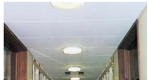
Figure 35 Suspended AIB ceiling tiles in a corridor
