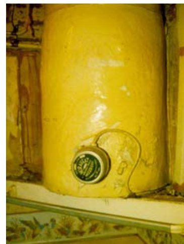
Figure 18 Domestic hot water cylinder lagged with asbestos
