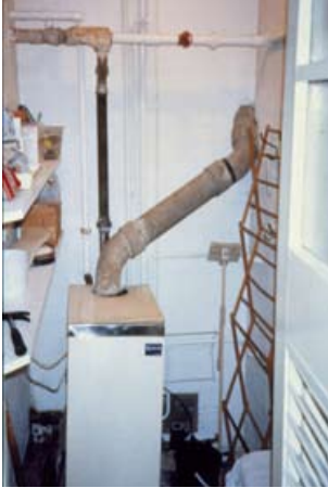
Figure 32 Asbestos cement flue on a domestic boiler
