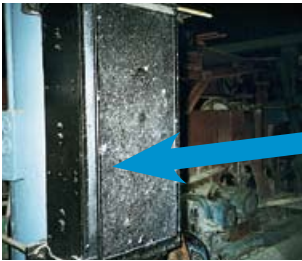
Figure 37 Asbestos debris on an electrical box, adjacent to a machine which was used to make bituminous roofing felt containing asbestos
