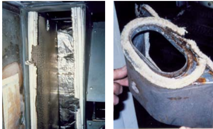
Figure 1 Asbestos paper lining Figure 2 Asbestos rope seal
