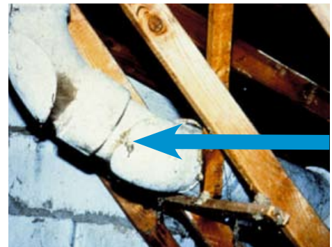
Figure 24 Asbestos cement flue in a ceiling void
