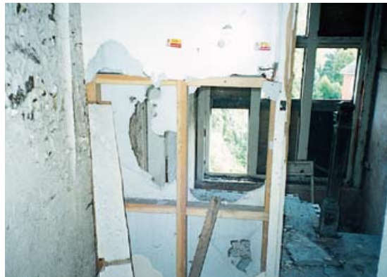
Figure 33 AIB wall panels badly damaged during poorly planned and uncontrolled work
