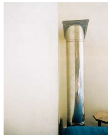
Figure 11 Metal/asbestos flue pipe – the asbestos is between the inner and outer layers of stainless steel
