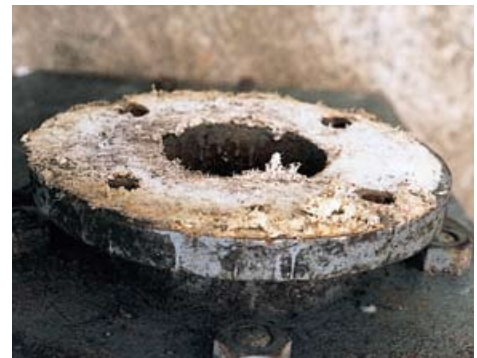
Figure 22 Debris from an asbestos gasket on a pipe flange
