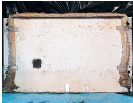
Figure 21 Asbestos rope seal and soft panelling on the burner/heat exchanger of a domestic boiler
