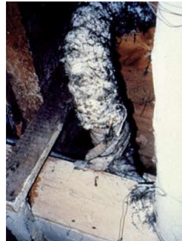
Figure 26 Asbestos rope pipe lagging
