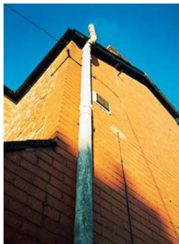
Figure 17 Asbestos cement flue – external
