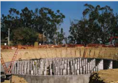
TreePeople Center Cistern, USA
