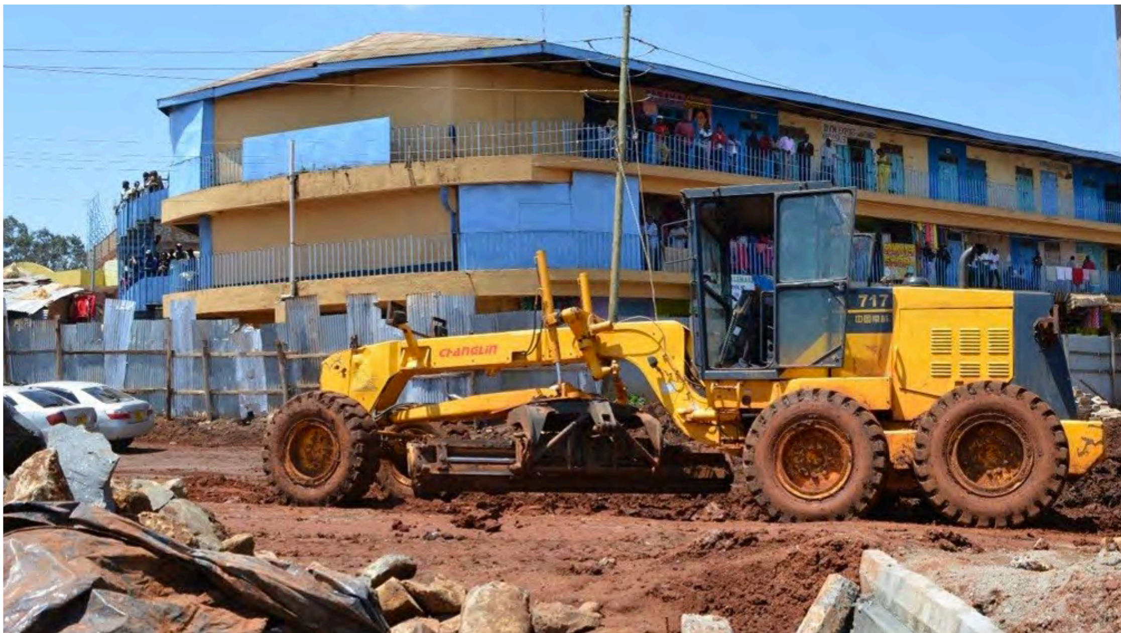
County road equipment constructing a bus station in Kitale, Trans Nzoia County
