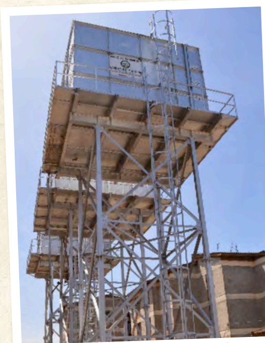
Highrise estate borehole and water collection tanks are helping ease water problems of residents.
