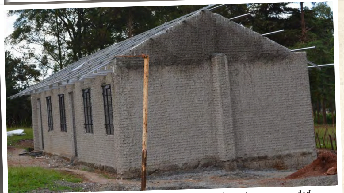
Soi Primary ECDE classrooms under construction using an expanded polystyrene system (EPS) in Trans Nzoia County.
