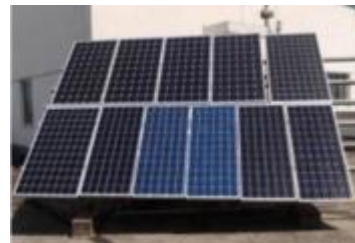
3. Outdoor test bed with different conditions.
