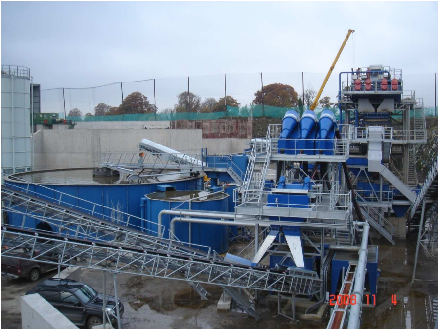
Static washing plant for recycling center facilities
