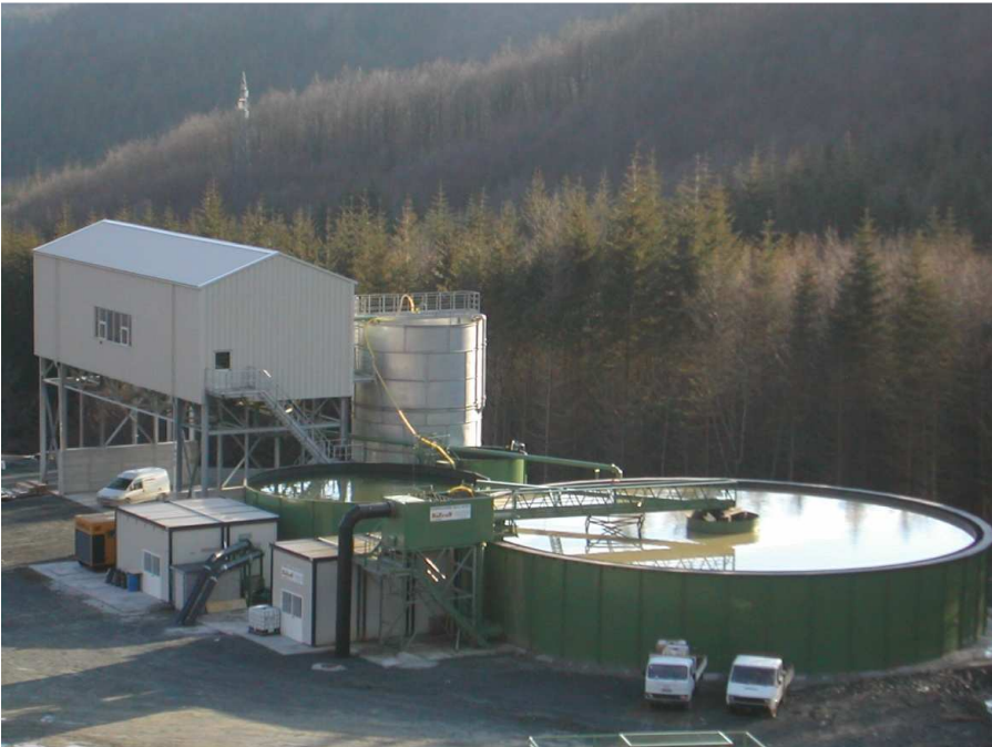
Water treatment and filter press plant
