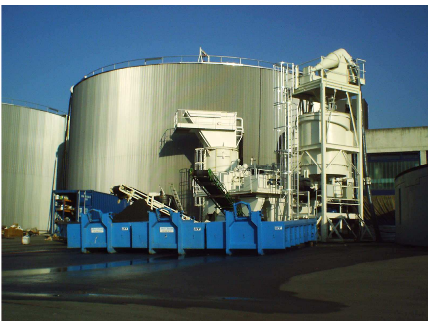
Sand & mud treatment for urban water treatment plants.
