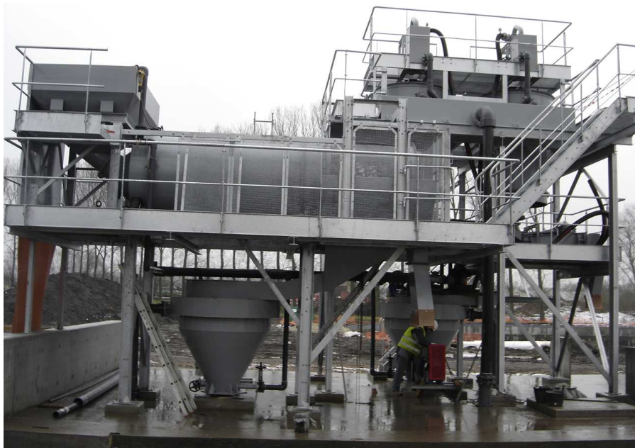
Sand washing plant for sewer collection
