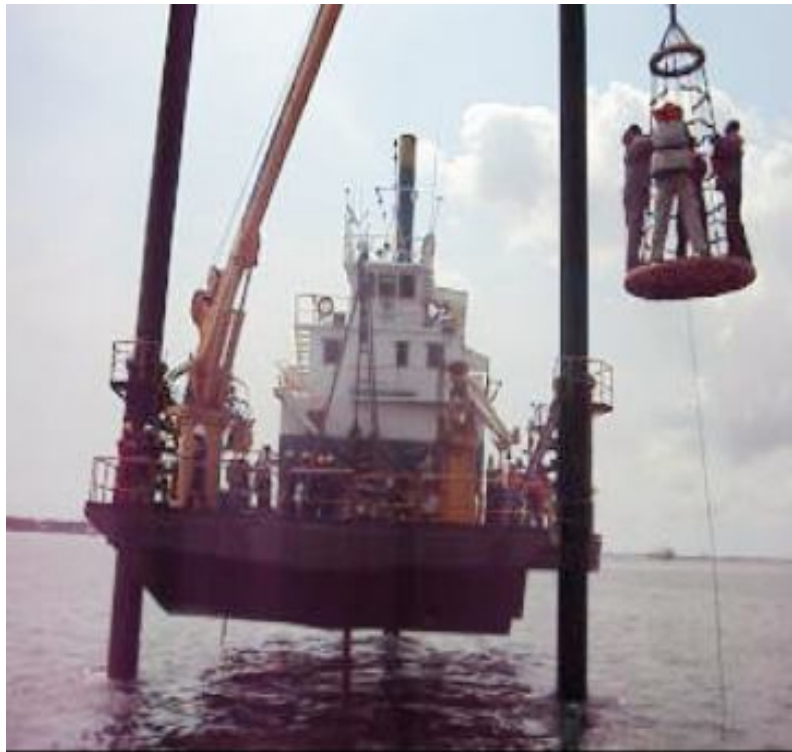
Deep soil investigations on a JACKUP barge at the suspension Bridge location on Bonny River: Visiting NDDC, Consultant staff and pressmen being lifted on to the barge at Ch. 196 + 250
