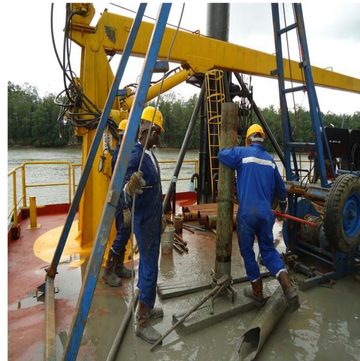
Deep soil investigation in progress on a JACKUP barge at bridge location of Andoni River at Ch. 179 + 110
