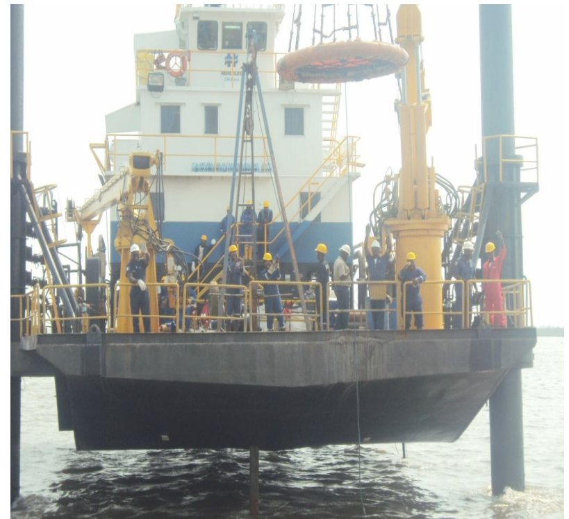
Deep soil investigations on a JACKUP barge at the suspension Bridge location on Bonny River at Ch.194 + 750
