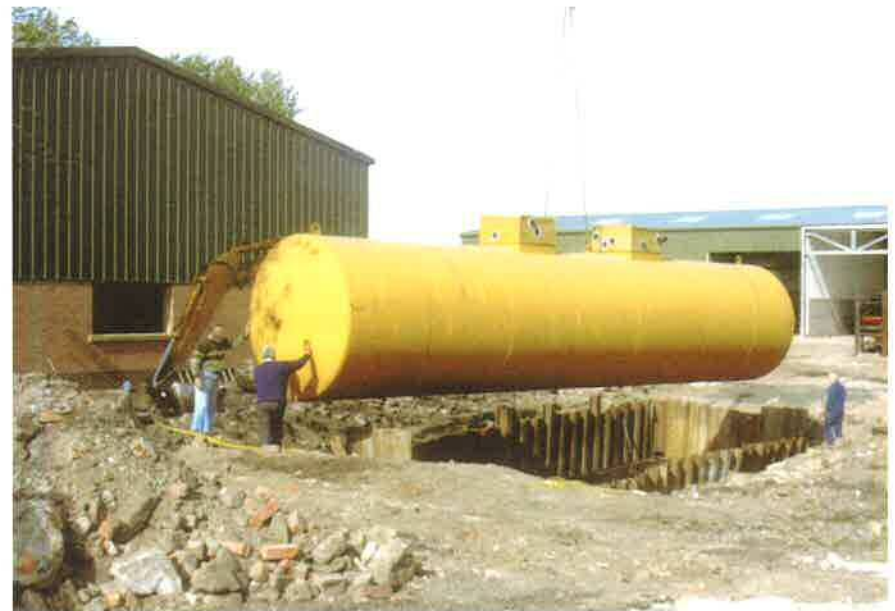
Andrew, Harry Boardman and Harry Wilkinson manoeuvring the diesel tank into place
