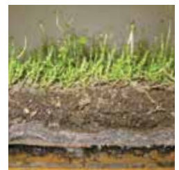
A section showing the different layers of an engineered green roof, from the base drainage layer to the upper vegetated layer (Photo by Tyler Carson)
