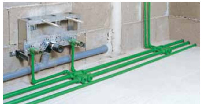
Floor distribution with distribution blocks
