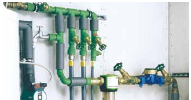
House connection station
