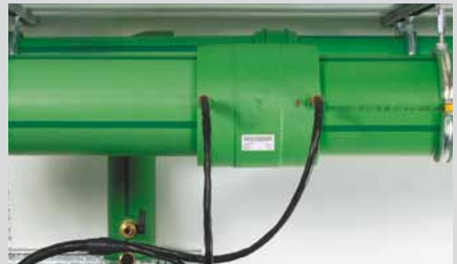
Adjust the socket diameter on the welding device. Start and control welding process. Keep the cooling time. Finished!
