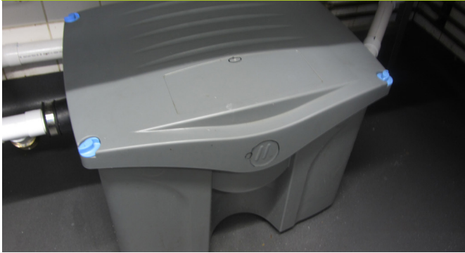
28 July 2017 - F.I.T unit connected to waste pipe of a double bowl pot sink and single rack dishwasher machine. No bio-dosing at this stage in trial.
