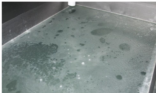
Grease in Mechline's skimmer tank waiting to be collected and weighed.
