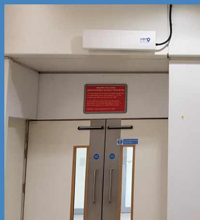
Reader fitted above doorway
