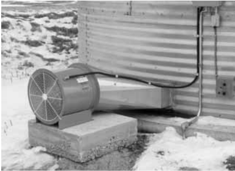
Figure 14: A photograph of an aeration unit which is attached to a grain silo (Canadian Agriculture, 2001).
