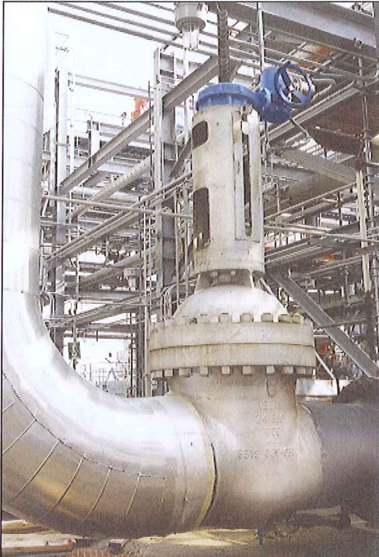
Carbon steel gate valve (ASME Class 600), used for boiler feed water installation at a Hydrogen Plant in Texas.
