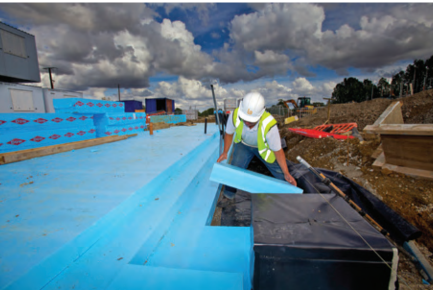
ABOVE: Insulation being installed below the floor slab Photo: DOW Building Solutions
