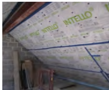
Internal view of a 'Cathedral' style roof under construction. Photos: Green Building Store
