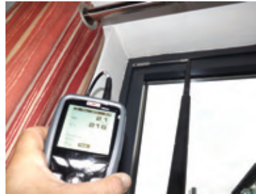
Extending vane anemometer showing a high air velocity of 2.1 m/s through a gap at the head of a balcony window
