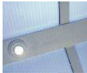
Lighting - integrated downlighting in the roof ridge space and pelmet surround.
