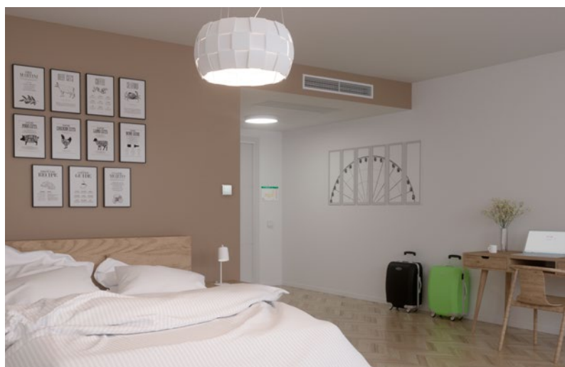
Hotel room with setpoint selector switch, waterborne cooling and heating as well as demand-controlled air. Key card holder for occupancy.
