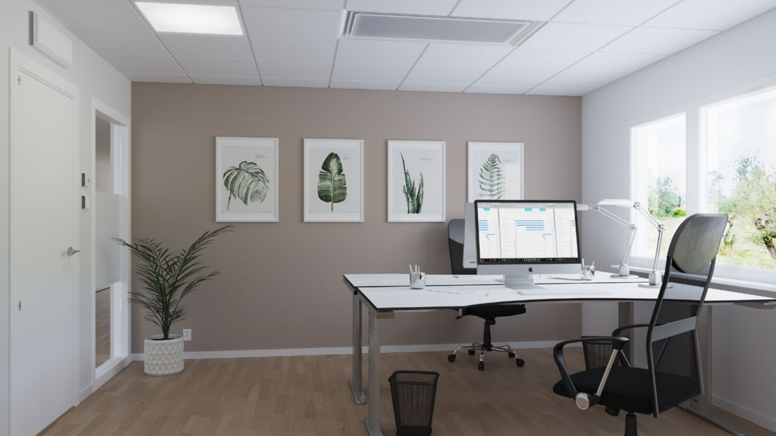
Waterborne office with setpoint selector switch and occupancy sensor for demand-controlled ventilation, cooling and heating.
