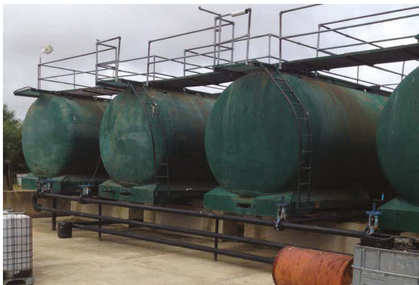
Figure 4.19 Lidsey Separation and Storage Tanks
