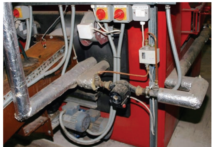
Figure 4.34 Connections to a water cooled grate showing cooling pump
