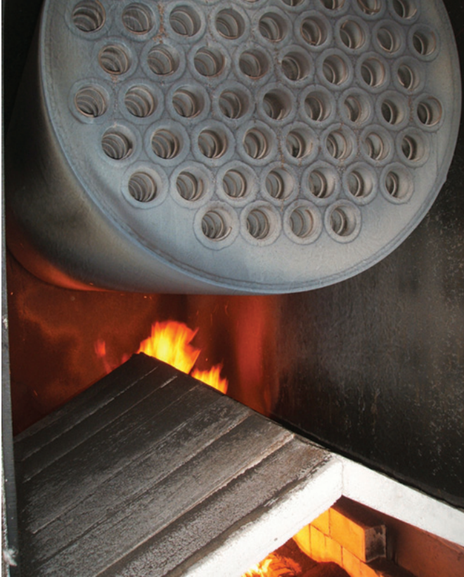
Figure 4.21 Arch of refractory lining above firebed with horizontal fire tubes at top
