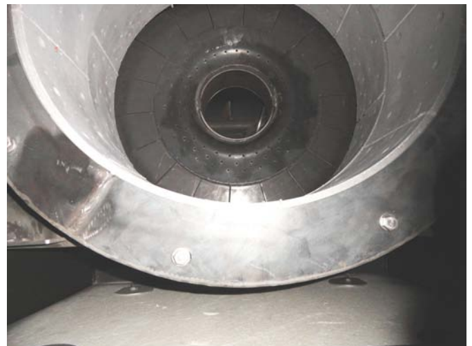
Figure 4.20 Cylindrical refractory lining in a 400 kW underfed stoker boiler showing fuel feed auger beneath grate, primary air holes in the grate and secondary air holes in the refractory
