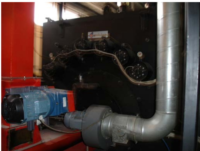
Figure 4.30 Exhaust gas recirculation duct and fan on a 1.5MW biomass boiler
