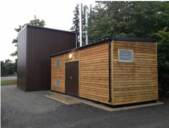
Figure 4.46 Packaged boilerhouse operating on woodchips (woodchip store on left)
