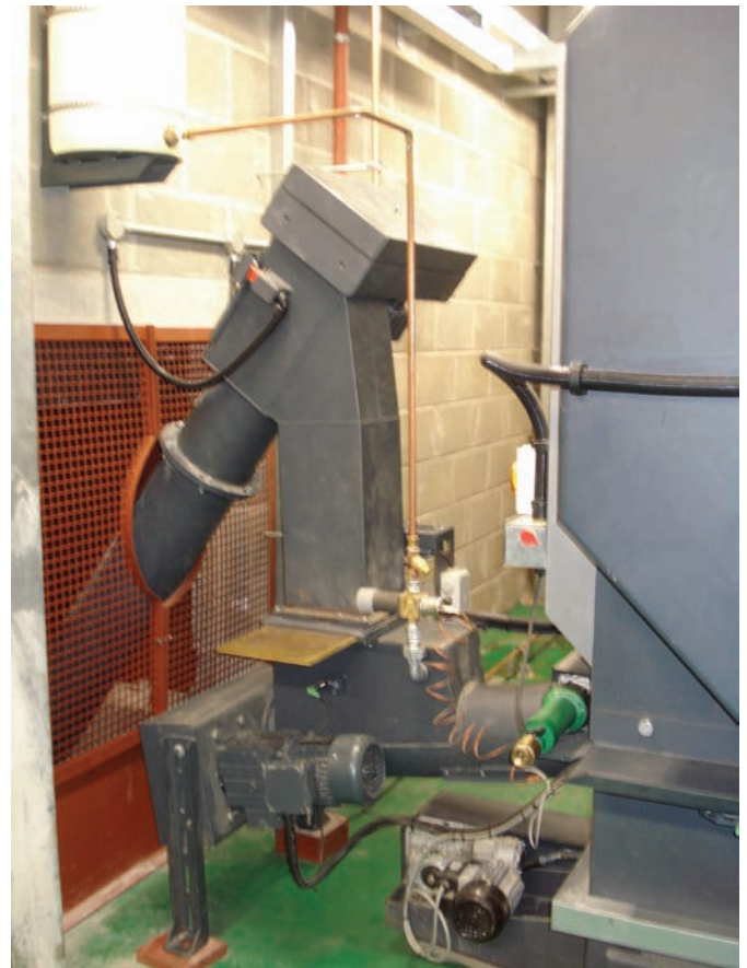
Figure 3.18 Water bottle and direct acting drench valve on fuel feed system
