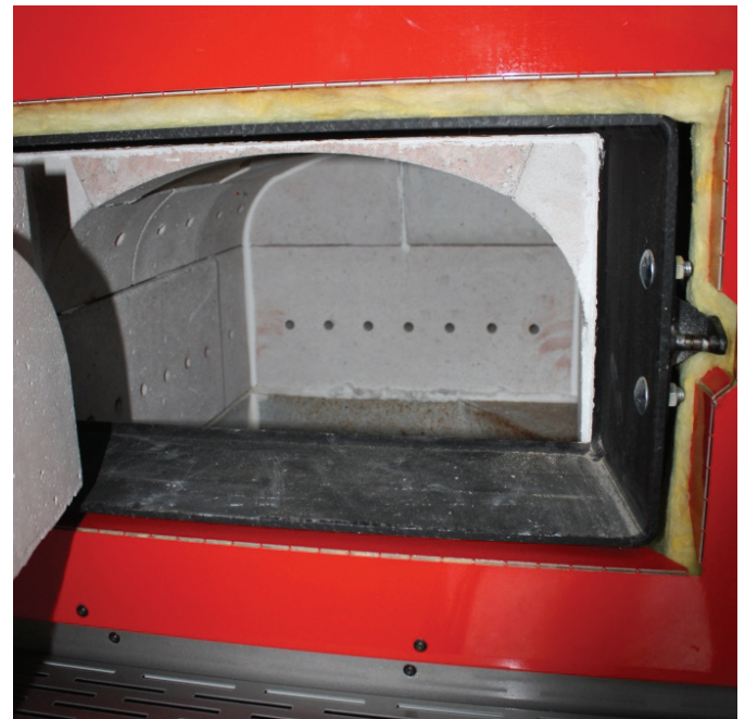
Figure 4.23 Refractory lining in underfed stoke boiler
