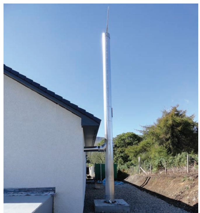
Figure 10.1 130 kW biomass boiler flue showing a lightning conductor
