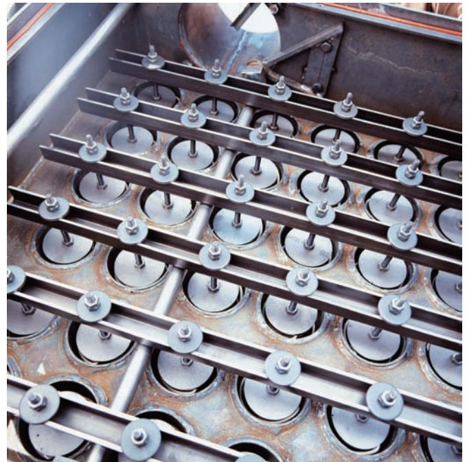
Figure 4.37 Turbulator shakedown mechanism on a vertical tube boiler
