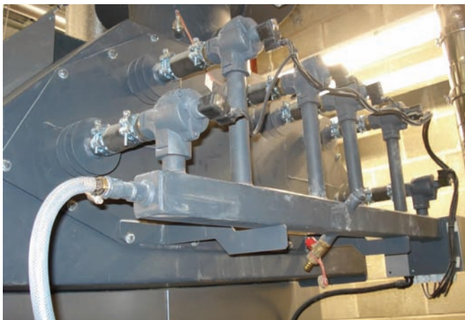
Figure 4.36 Compressed air cleaning nozzles on a horizontal tube boiler
