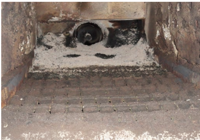
Figure 4.5 Stepped grate in an overfired stoker boiler
