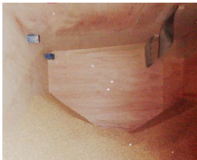
Figure 3.13 Internal view of pellet store, showing fuel fill pipes (left) and pellet impact mats (right)
