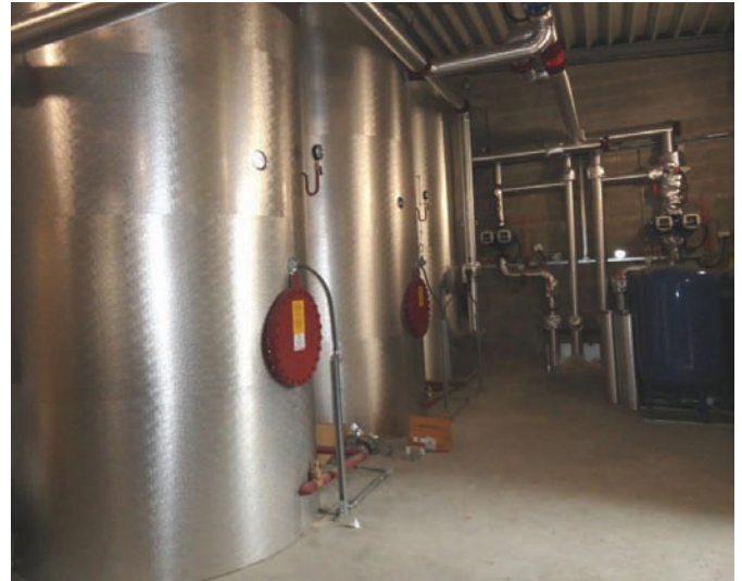
Figure 5.1 Three 10 000 litre thermal stores on a 400 kW biomass system
