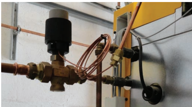
Figure 4.25 Emergency heat exchanger pipework with direct-acting valve and temperature probe sensor withdrawn from its pocket
