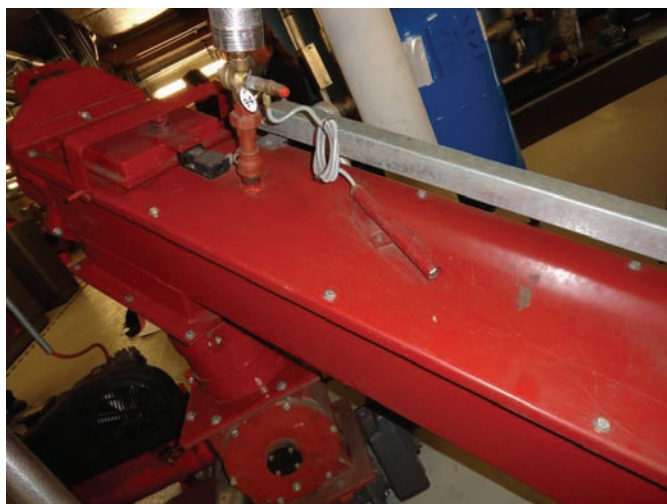
Figure 3.17 Mains water drench valve with flap valve housing below
