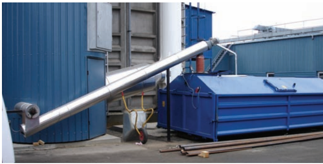
Figure 4.35 External ash bin on a 3 MW biomass boiler
