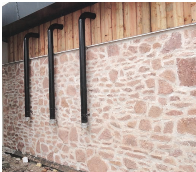
Figure 3.11 External view of wood pellet fuel fill and pressure relief pipes
