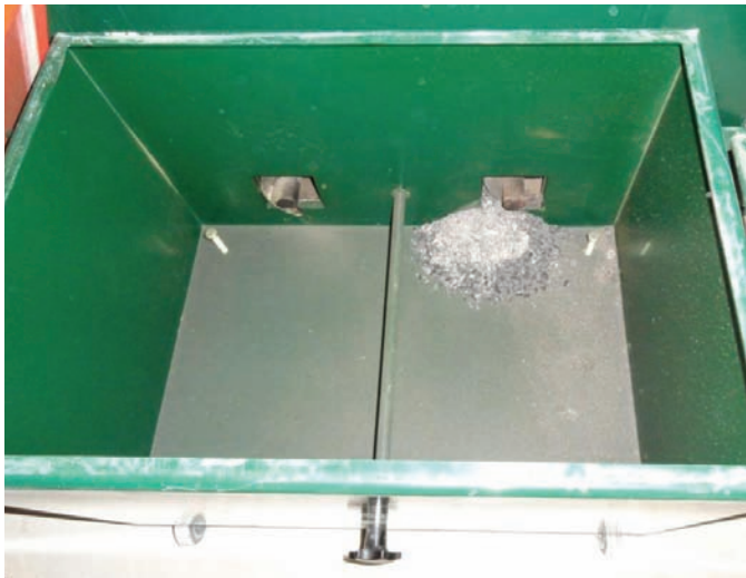
Figure 2.7 Ash from a newly commissioned 400 kW boiler operating for 12 hours (100 mm across)
