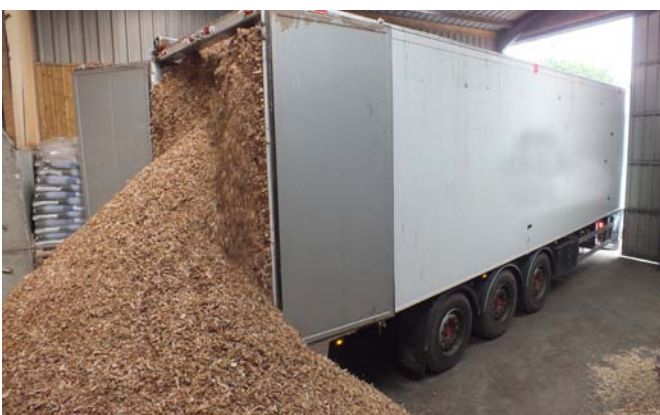
Figure 3.7 Woodchip fuel delivery from a walking floor trailer
