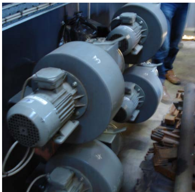
Figure 4.28 Primary combustion air fans on a 2 MW overfed stoker boiler
