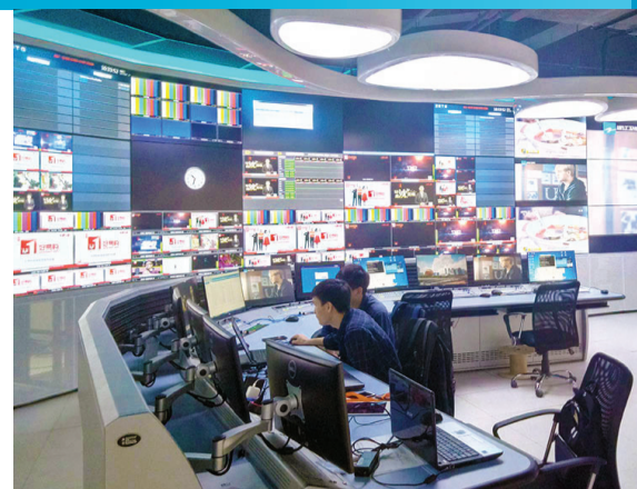
Zhejiang Radio and TV Group has employed IHSE's Draco tera KVM switch to connect 100 operators to more than 70 source devices via Cat X or fibre cables in its new Zhejiang International Film and TV Centre building.
