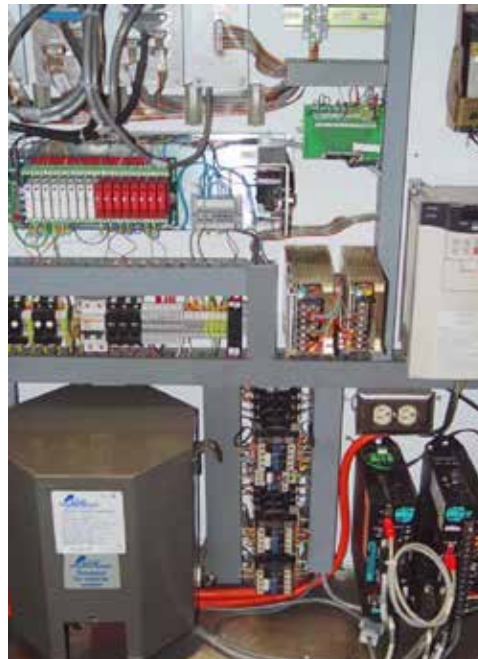
Actual BH8000S main control cabinet with new registration controls upgrade installed.
