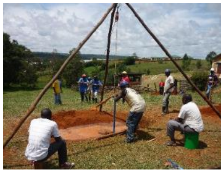
Above: Manual drilling training at the SHIPO SMART Centre, Tanzania (H. Holtslag) [098]
