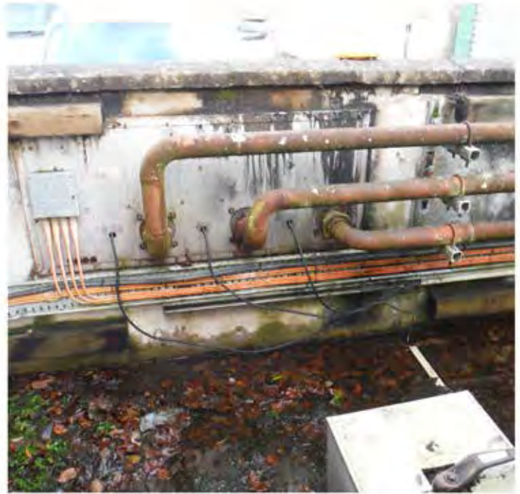
Unsealed & ineffectively sealed cable & pipe entries into the bund
