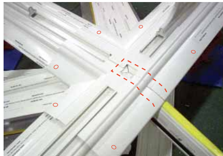
Position the 2 covers onto the joint over the lines of sealant. Compress the joint and rivet the covers to the ridge top caps in the 6 positions shown. Use the plastic rivets provided through 5mm diameter holes.
