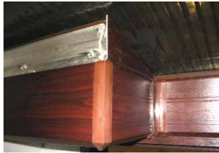
Extra box gutter under clad is supplied to cloak of the remaining raised leg section.
