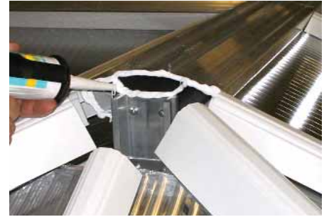
Remove the bung and silicone seal around the ridge profile making sure the silicone runs down to the glazing level on both sides.
