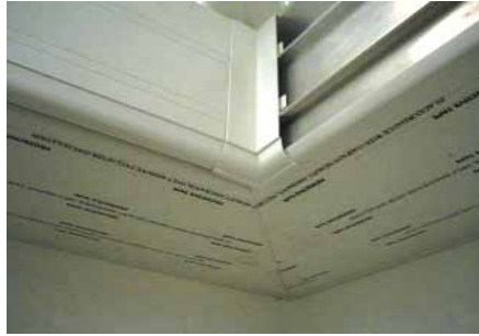
Fit the box gutter side clads in the same manner as the internal eaves beam clads.
