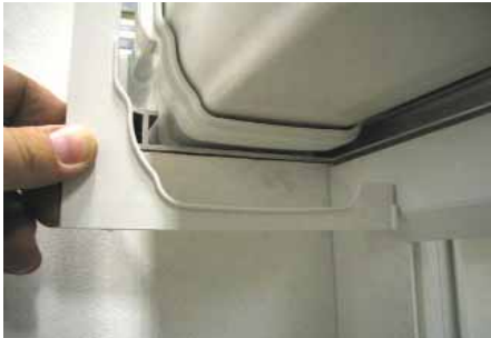
The box gutter end cap can now be installed. On some roof designs this may need trimming to suit.
