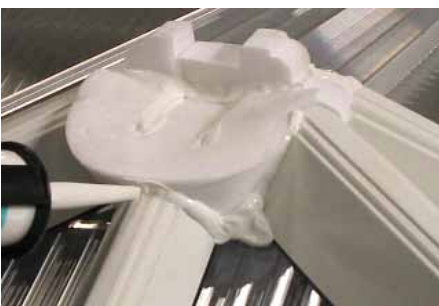
Finally run a continuous seal around the foam bung so it is sealed to the glazing and rafter top caps.
