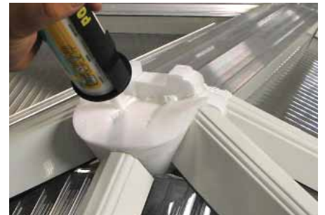
Silicone seal the joint between the two foam bungs including the joints between the two v-notches.
