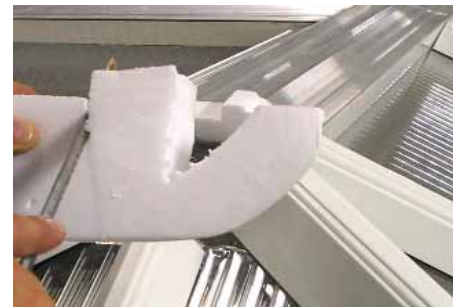
If the bung is too large for the aperture, cut two v-notches in to the bung using a hacksaw blade.
