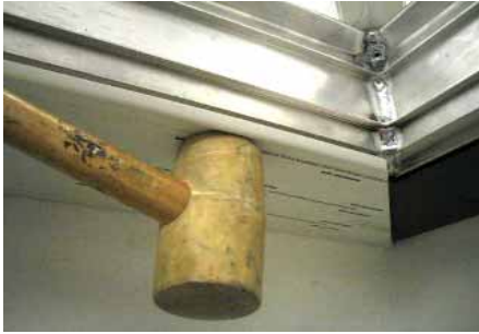
Box Gutter: Position then knock the box gutter under clad in to position using a rubber mallet.
