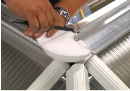
Some corner ridges will have a radius end detail. Cut the foam bung components down to fill the void.
