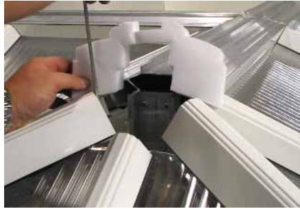
Using a hacksaw blade cut down the width and height of the bridged section of foam bung so that it fits snugly between the rafter top caps and finishes level with the top of the ridge.
