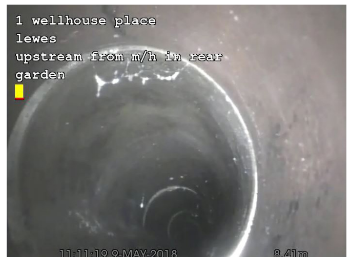
The sewer remains clear, 2 years after GreasePak first installed, May 2018.
