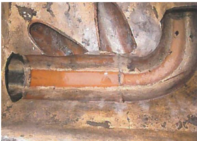
The clear sewer run at the end of the year-long trial, April 2017.
