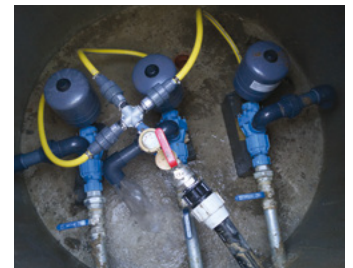
3 Papa Pumps with delivery ports connected to one delivery pipe.
