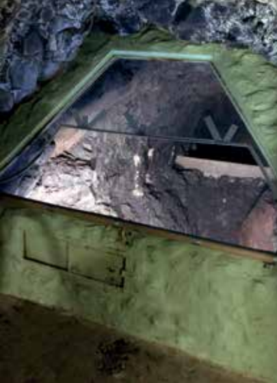
Original portal window looking into the water aquifer below. (Note that this view does not clearly show the badly deteriorated window structure.)
