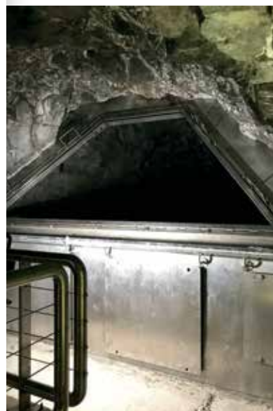
New 316 stainless steel viewing portal
