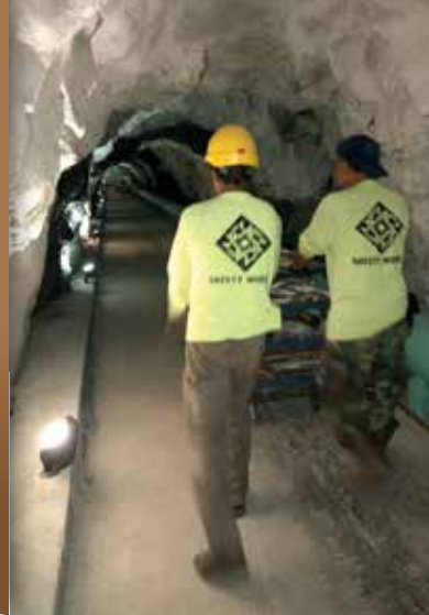
CMC workers transport the deteriorated window structure through a tunnel to the elevator.
