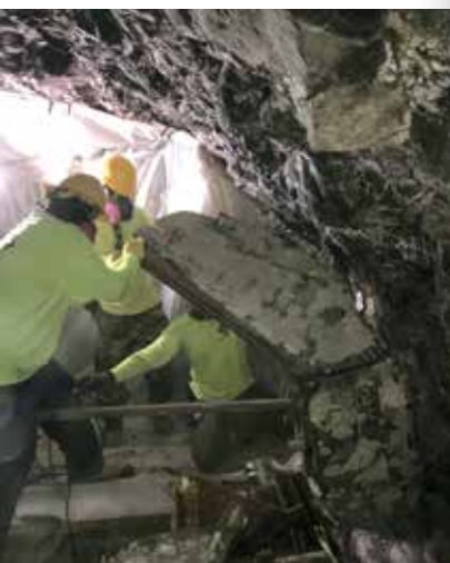
CMC's crew members remove the badly deteriorated window structure. (Note containment to protect the water source in the background.)
