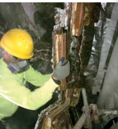
After installing containments, Civil-Mechanical Contractor crews begin the tedious task of removing the window structure, piece by piece.
