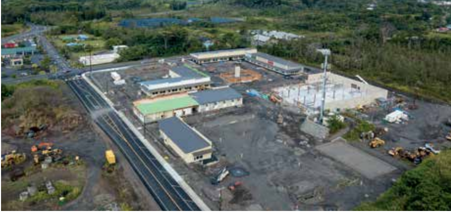
Meridian Pacific's construction of Puna Kai Shopping Center in Pahoehoe continues on schedule. PHOTO COURTESY HAWAII AERIAL VISIONS LLC
