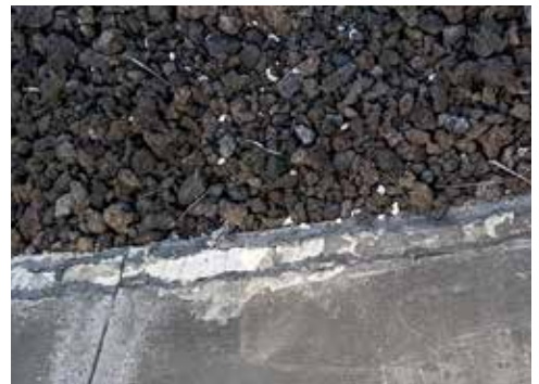
Spalling walkway at a beachside resort PHOTO COURTESY ALOHA MARKETING LLC
