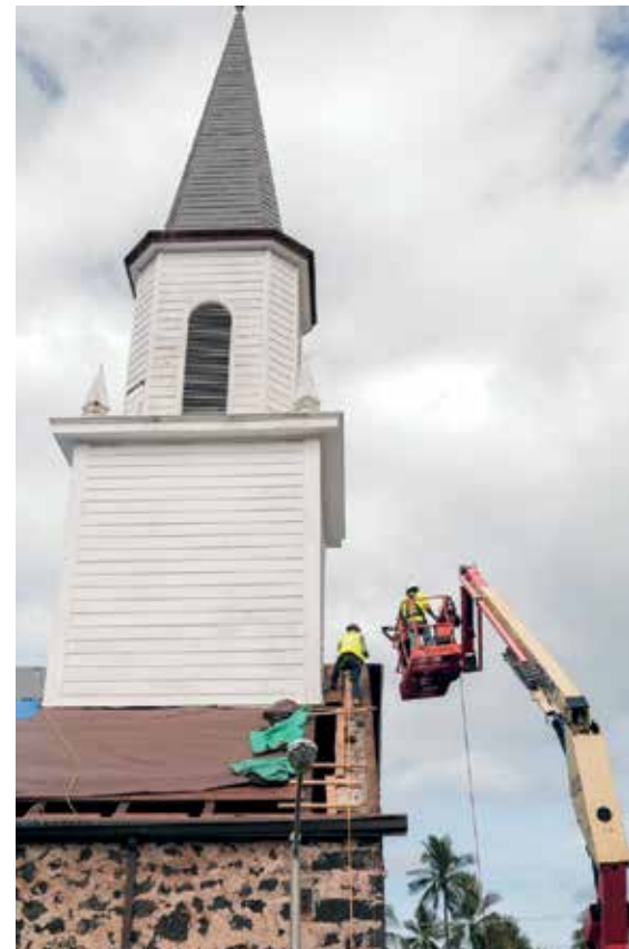
Alii Builders continues preservation work on Mokuaikaua Church in Kailua-Kona. PHOTO COURTESY LOGAN PENROD
