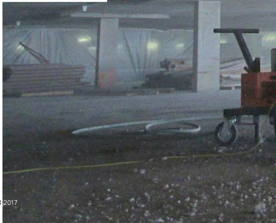
Typical parking structure deterioration.
