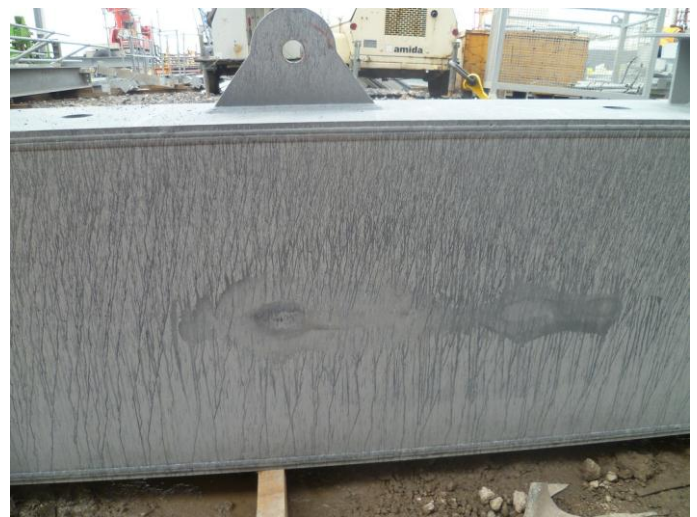
One of the beams after it rained on site showing oxide streaks
