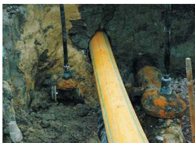
Fig 6-3: Pulling in an egeplast SLM ® DCT gas pipeline under adverse soil conditions
