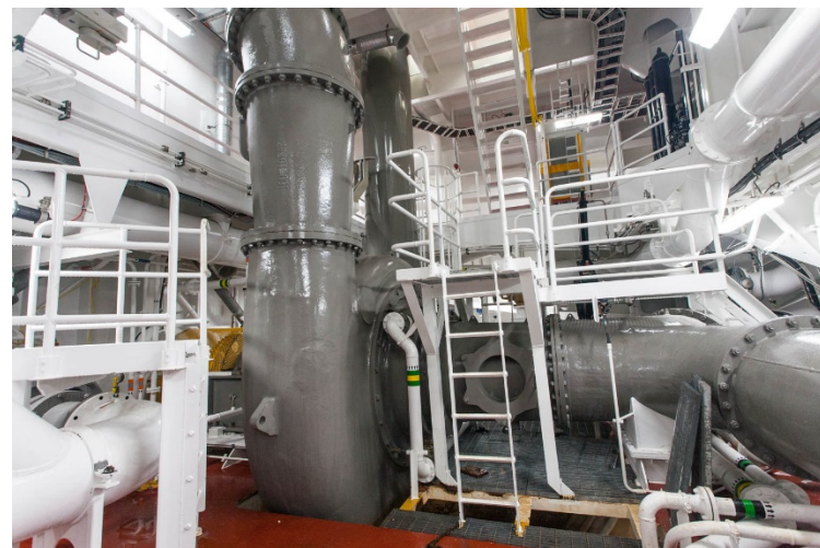
Dredge Pump Room
