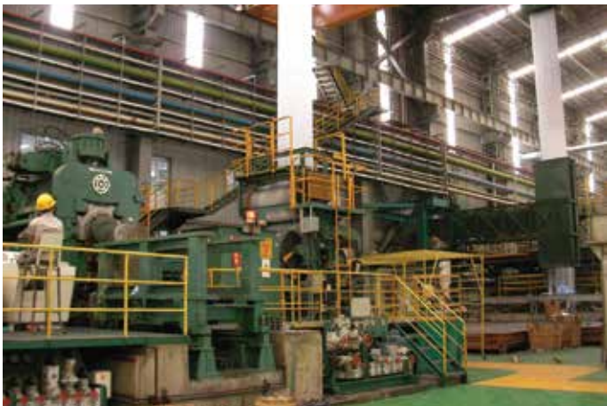
No.1 Continuous Galvanizing Line
