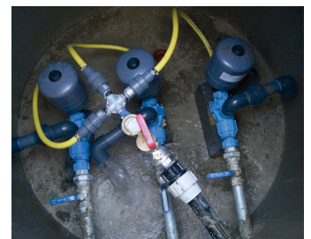
3 Papa Pumps with delivery ports connected to one delivery pipe.
