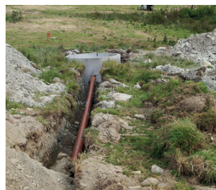
Installing the supply pipe from the supply tank to the pump chamber.
