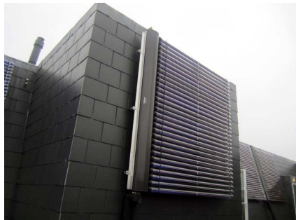
Thermal solar panel
