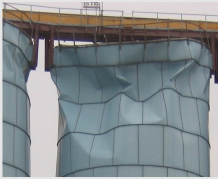
Damage due to improper design
