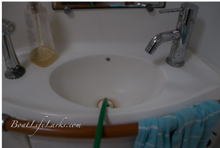
Brine goes overboard through the drain in the head.
