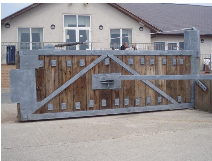
Another view of the tide-gate, showing the locking bar
