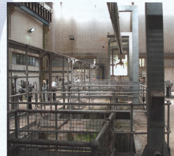
The Bosker installation at Thames Water's Deephams WWT works serves several inlets
