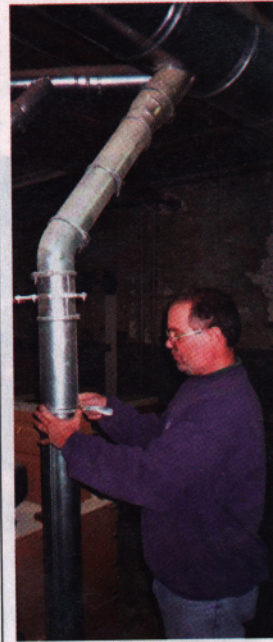
The company's Torit dust collector is fed by snap-together ductwork by CDM. Carmen Vona says it allows quick hooking and unhooking of equipment to and from the system.
