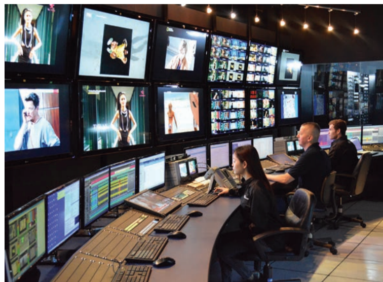
ABS has master control rooms located in the Philippines, Indonesia, and with its partner teleport in Hong Kong, to manage and operate broadcast services for its clients in the media industry.
