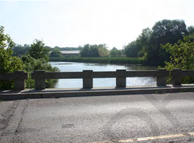
Figure 6.8 The Brock Street South's Pringle Creek Bridge requires an additional pedestrian walkway along it's western edge
