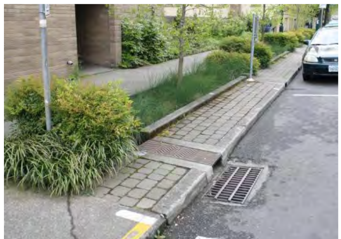
Figure 3.17 Hardscaping should be carefully combined with adjacent landscaping treatments to reduce the impacts of stormwater runoff (bioswale in Portland, Oregon).
