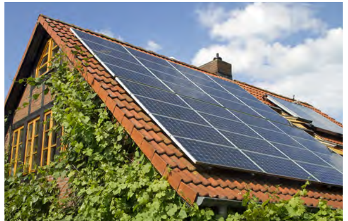
Figure 3.40 Roof mounted photovoltaic panels can offset energy use and provide energy if local grid is unavailable.
