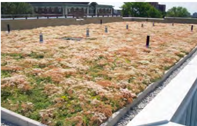
Figure 3.51 Green roofs are lower maintenance and more durable as the roof membrane is protected (ESRI Canada Ltd. rooftops, Toronto)
