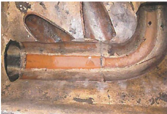
The clear sewer run at the end of the year-long trial, April 2017.
