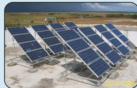
Solar Panel Arrangement
