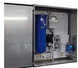
60 lit/min system in an enclosure
